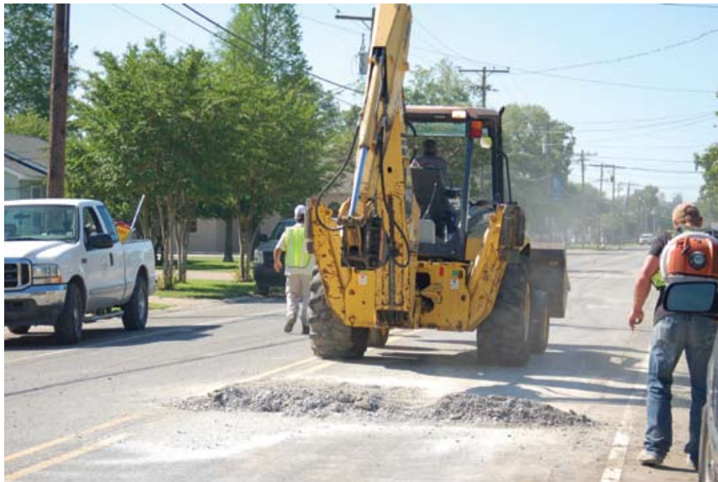
Road work like the construction on North Jefferson Avenue is part of the construction to upgrade the sewer collection system in Port Allen. Crews are lifting the road to reach the lines, which bring waste water to the sewage facility. There are 59 points on local roads impacted by the work.
