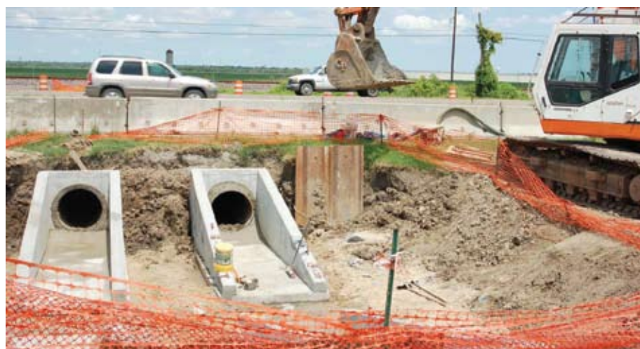
DRAINAGE PROJECT CONTINUES... A drainage improvement project that includes installing two huge drain pipes under La. Hwy. 1 near Wal-Mart is well underway. The Louisiana Department of Transportation and Development is handling the project, which is part of the comprehensive plan to improve drainage in the area from Brusly to the Intracoastal Waterway. Parish President Riley "PeeWee" Berthelot said this drainage project and one already completed in the Lynndale area off La. Hwy. 1 should significantly improve drainage in that area.
