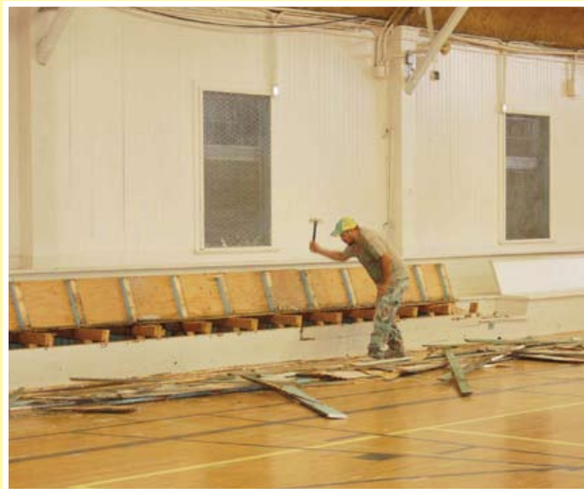
WORK UNDERWAY ON PORT ALLEN COMMUNITY CENTER... The Port Allen Community Center is now closed for public use during the renovation of the facility, which began in July. The $450,000 facelift includes a new side entrance, addition of a lift door at the back, removing bleachers (shown above) and dressing out the walls with wood wainscoting, replacing flooring and lighting and repainting. The project is expected to be completed by November 1.
